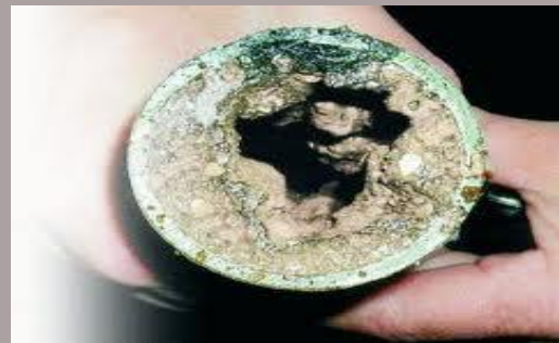
Plugged pipes with grease and food particles.
